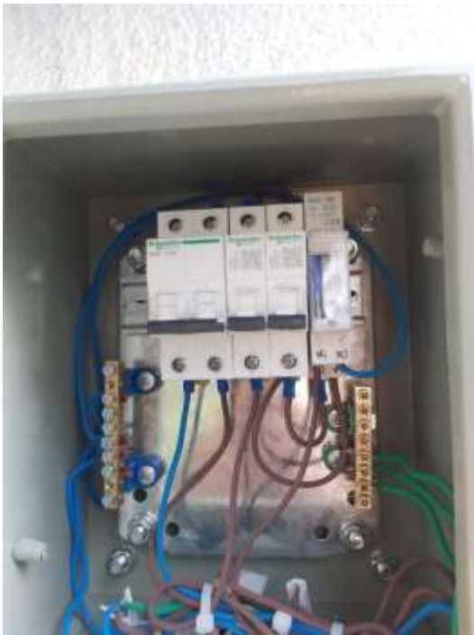
Figure A.12 Electrical box
